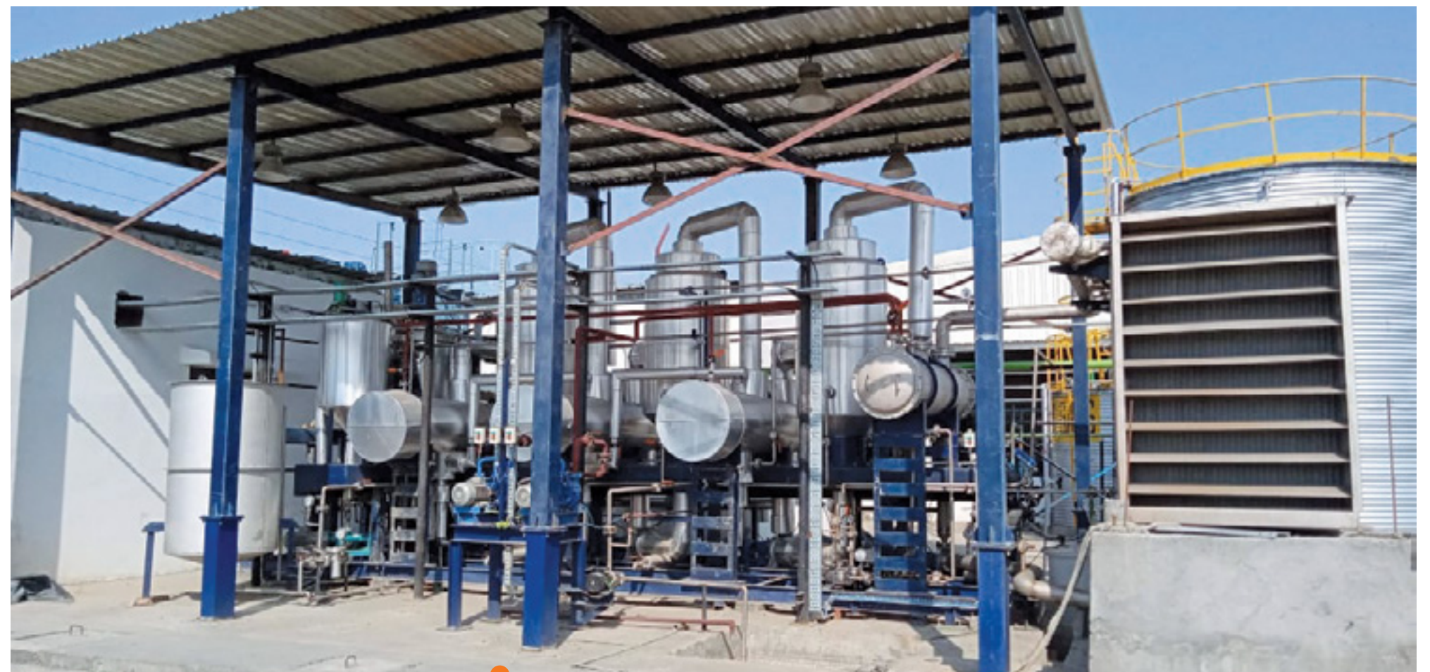
Zero Liquid Discharge (ZLD) Effluent Treatment Plant
